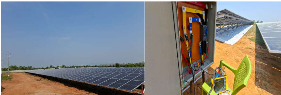
Fig.1 Snapshot of Solar panel and the recording of the data at the panel board using Power Quality Analyzer
